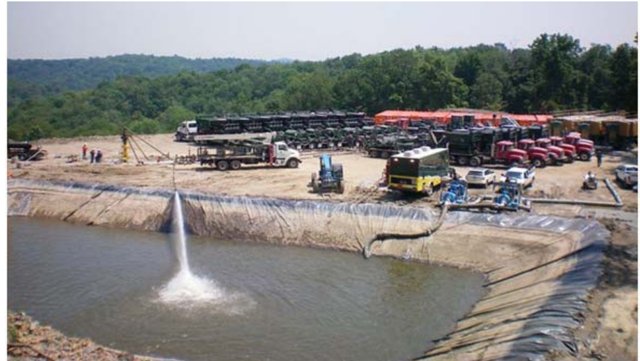
Lined impoundments provide temporary storage for water needed for hydraulic fracturing. (NETL's E&P Focus Newsletter )
