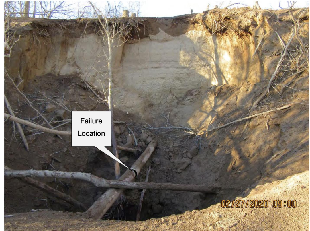
Figure 6. Failure Location (Upstream to Downstream)
