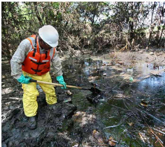
A contractor works to remove oil pools left after a spill from a refinery in Coffeyville, Kansas, contaminated floodwaters of the Verdigris River in 2007. Image Credit: Leif Skoogfors/U.S. Federal Emergency Management Agency. 15
