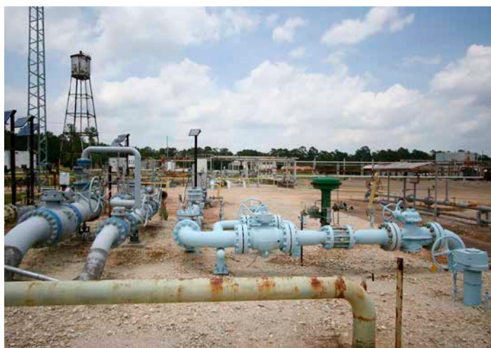
Natural gas infrastructure includes a large number of valves and connectors, such as at this gas processing facility in Montgomery County, Texas. Components such as these may be sources of gas leaks. Image credit: Roy Luck, Flickr. 12
