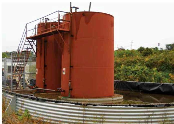
Storage tanks for produced water from natural gas drilling in the Marcellus Shale of Western Pennsylvania are surrounded by spill-containment structures. Storage tanks are one of the main sources of oil- and gas-field spills. Image credit: Doug Duncan, U.S. Geological Survey. 12
