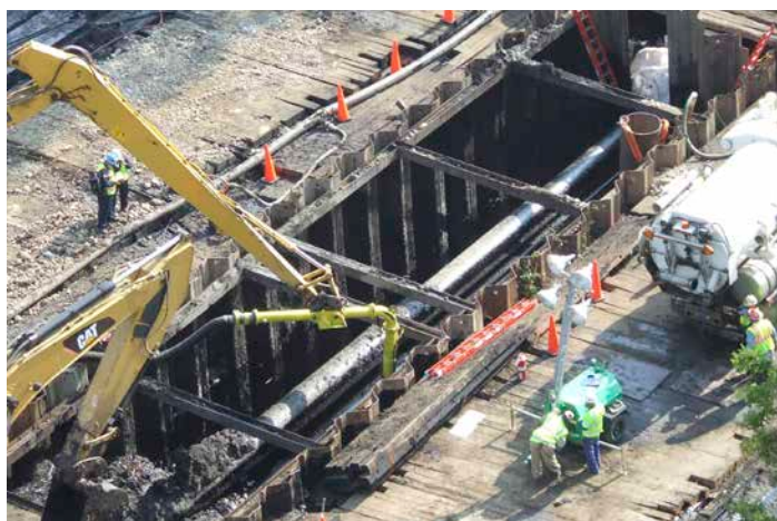
The damaged portion of Enbridge Line 6B is prepared for removal, having spilled hundreds of thousands of gallons of heavy crude oil near Marshall, Michigan, in July, 2010. Image credit: U.S. Environmental Protection Agency. 32
