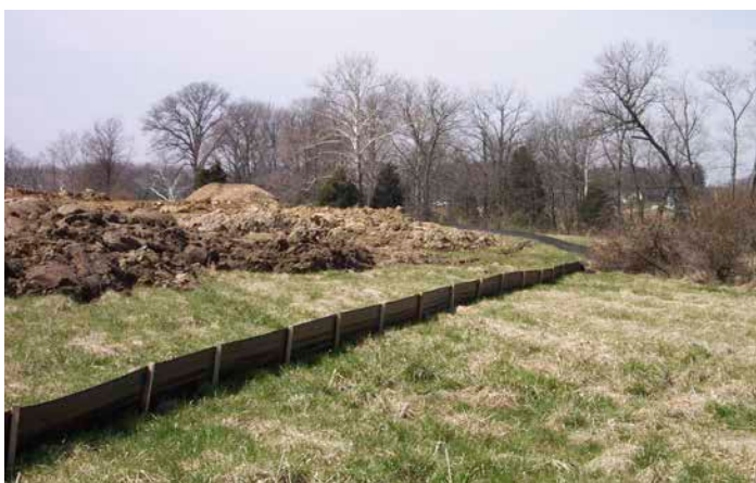
Plastic fencing to control soil erosion and stormwater runoff at a construction site. Image Credit: U.S. Environmental Protection Agency. 30
