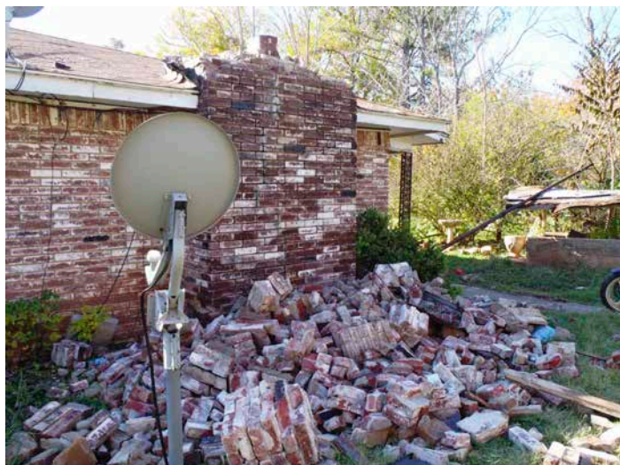
Damage caused by the magnitude 5.7 earthquake near Prague, Oklahoma, November 6, 2011. Unreinforced stone and brick buildings (especially chimneys) are some of the most vulnerable structures in any earthquake. Image credit: Brian Sherrod, USGS 10
